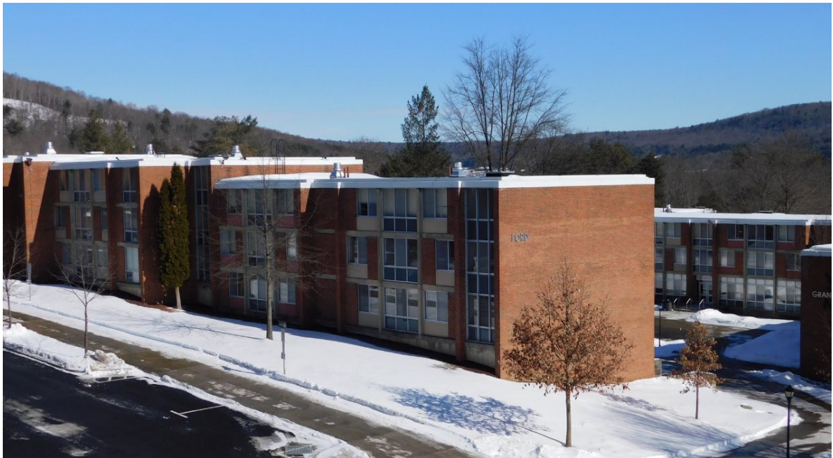
Ford Hall – Full renovation expected to occur from spring 2023 through summer 2024; building envelope, high efficiency HVAC systems, solar thermal domestic water; and designed to achieve SUNY goals for Deep Energy Retrofits (DER)
