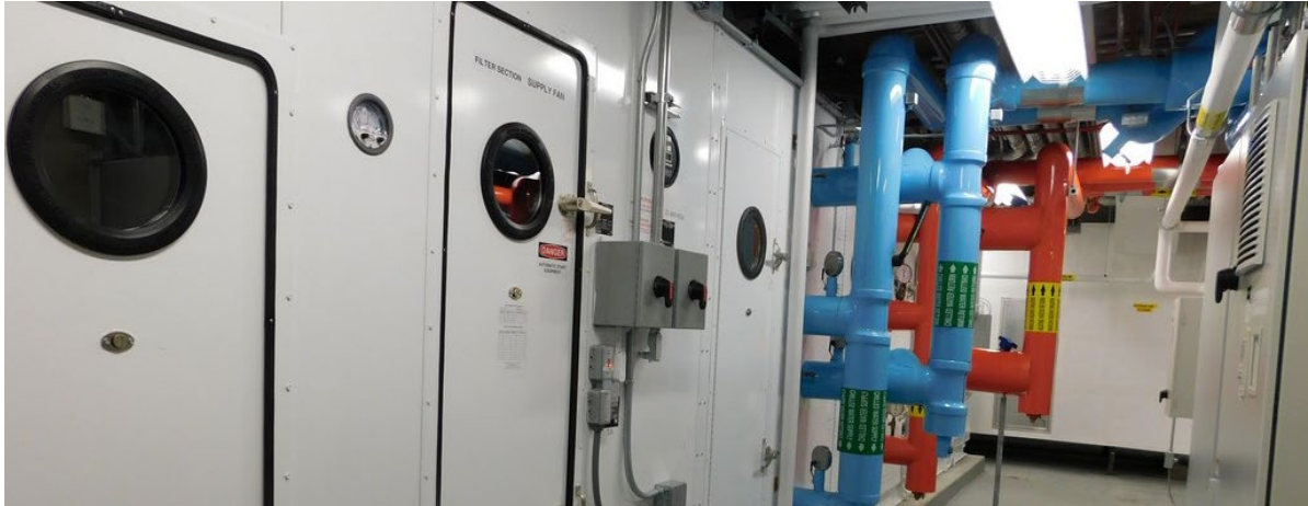
Physical Science II Building - Air Handling Unit #2
